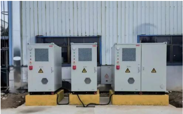
675kW/2088kWh Jiangxi Lesheng Synthetic New Materials Energy Storage Project
