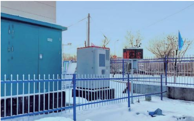
2.9MW/6.23MWh Xinjiang Yining Optical Storage, Charging, Swapping and Discharging Integrated Project
