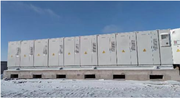
15MW/60MWh 100MW Photovoltaic Power Generation Project with Energy Storage in Dongle North Beach, Shandan County
