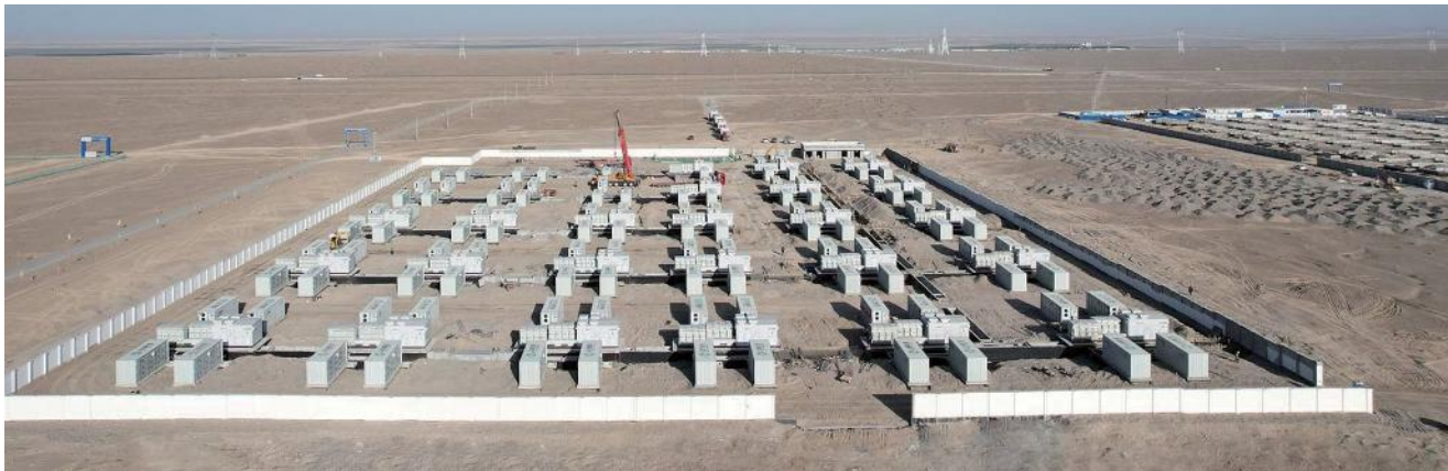
200MW/800MWh Limin Xinfeng County Independent Energy Storage Project
