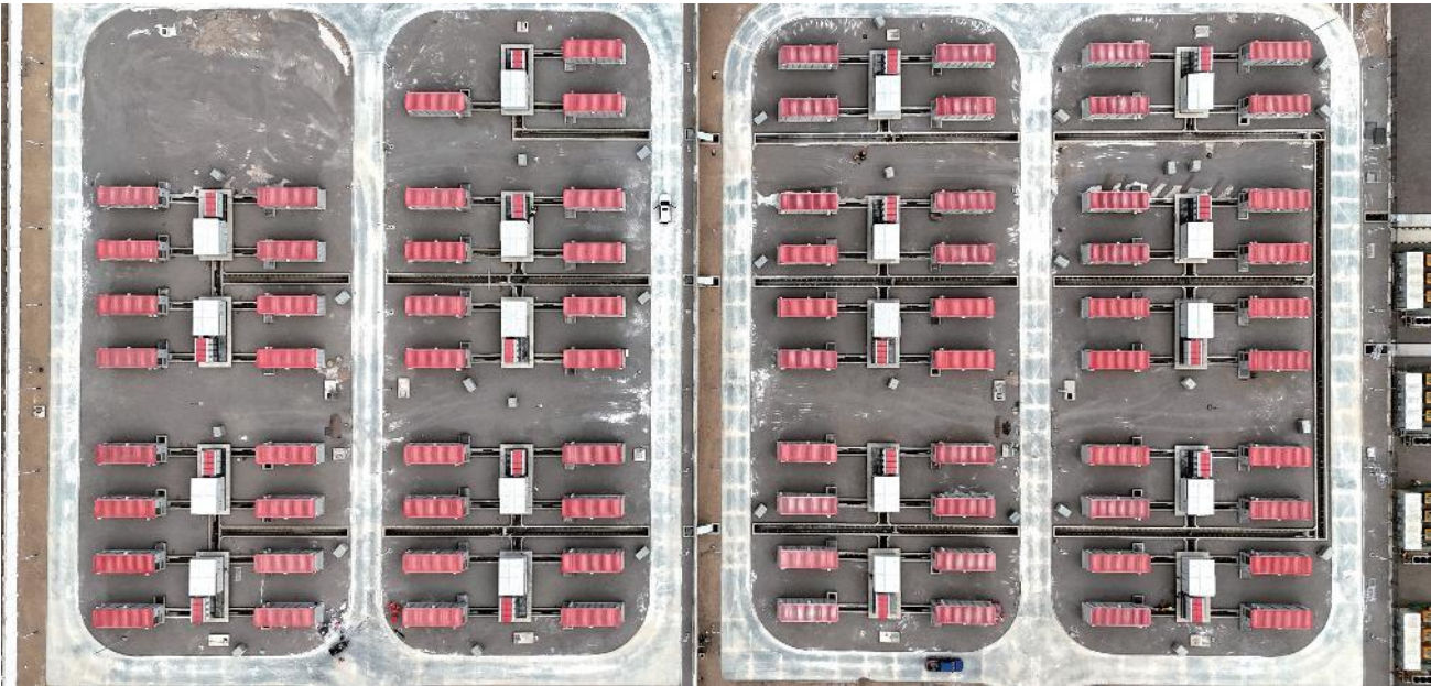
125MW/500MWh CNNC Xinyuan Xinjiang 1,000,000 kW Wind Power Source-Grid-Load-Storage Integration Project
