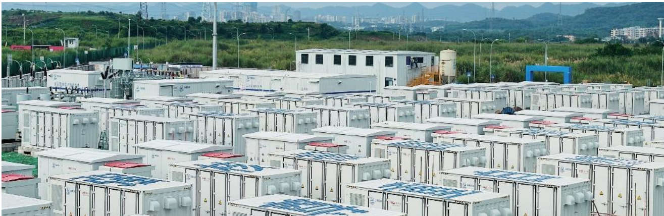
100MW/200MWh CNNC Huineng Chongqing Xiyong Comprehensive Bonded Zone Energy Storage Power Station
