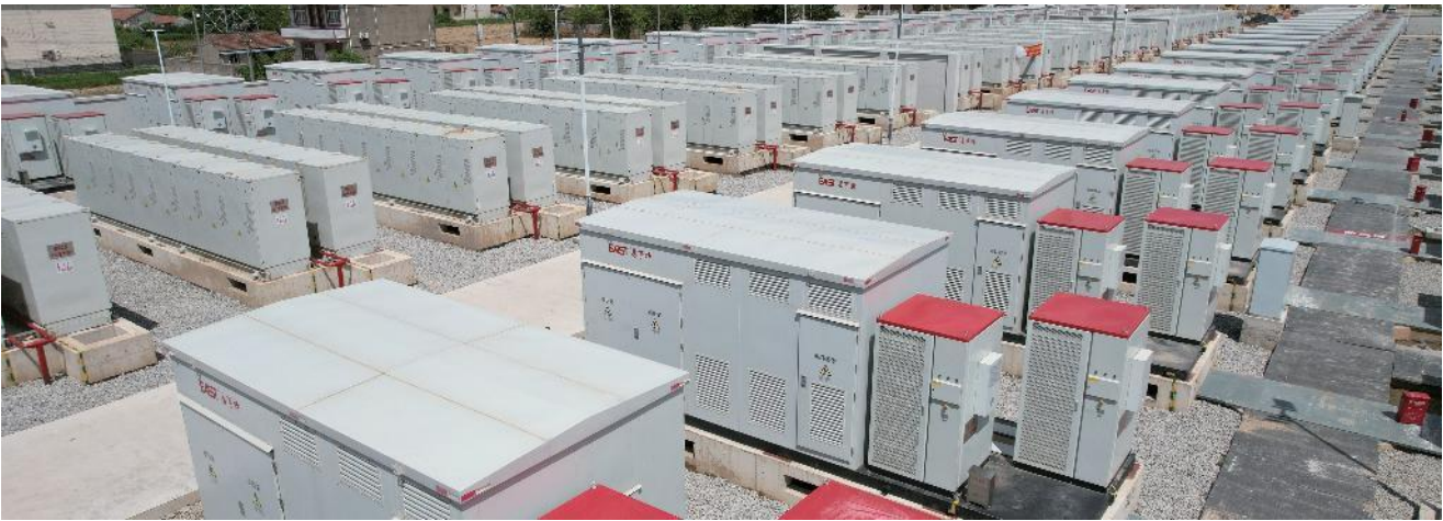
155MW/369.52MWh East Qidong Energy Storage Power Station
