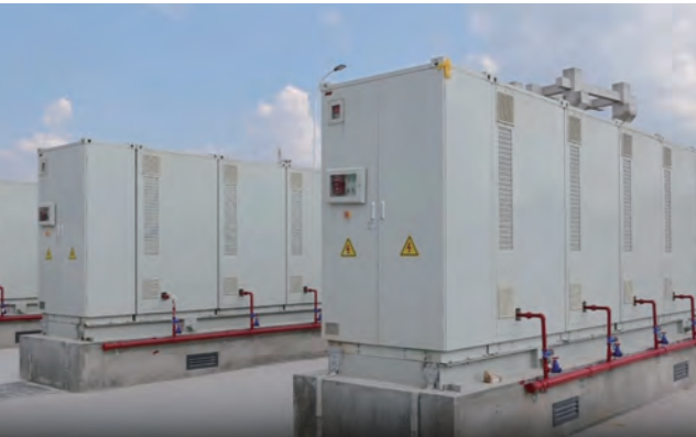
4.95MW/10.07MWh Zhejiang Sanmei Chemical User-Side Energy Storage Project
