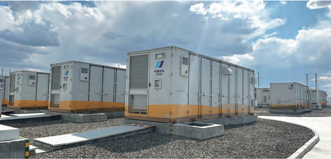
300MW/1200MWh Xinjiang Huadian North Tianshan Foothill Base 6.1 GW New Energy Project
