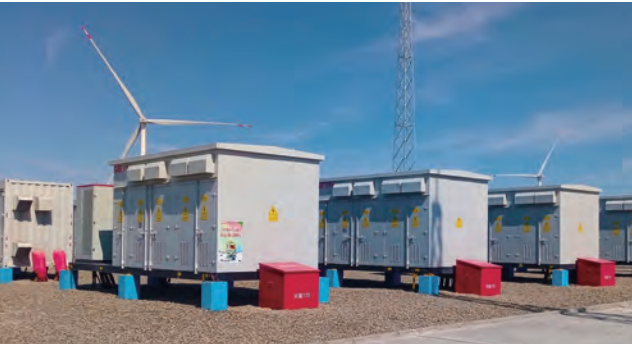
10MW/20MWh Energy Storage Matching for the 100MW Wind Power Project at Sishigejingzi, Mulei, by Changji State-owned Investment Xinneng
