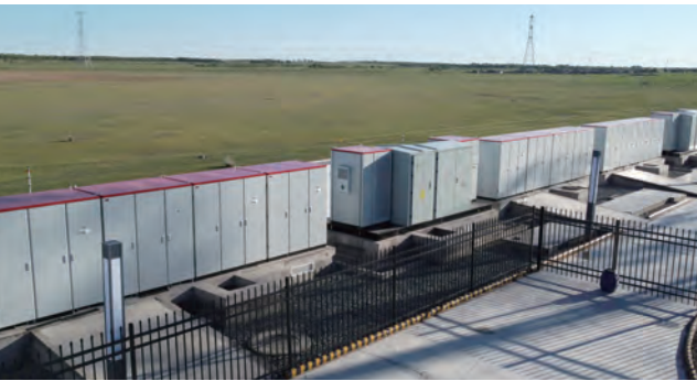
5MW/5MWh 100MW Energy Storage Supporting Project of the Kangbao Smart Microgrid Demonstration Project
