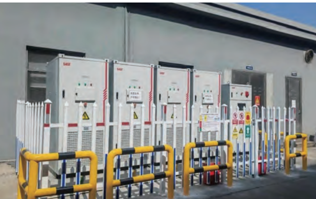
3MW/6.99MWh Zhejiang Yuhuan Suqiangge Industrial and Commercial Energy Storage Project
