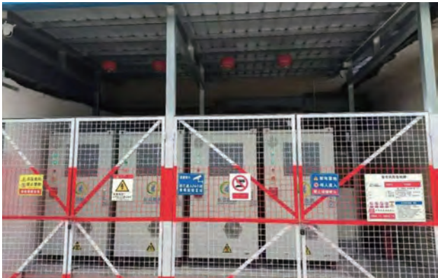
540kW/1044kWh Dongguan Energy - Dongling New Building Materials Energy Storage Project
