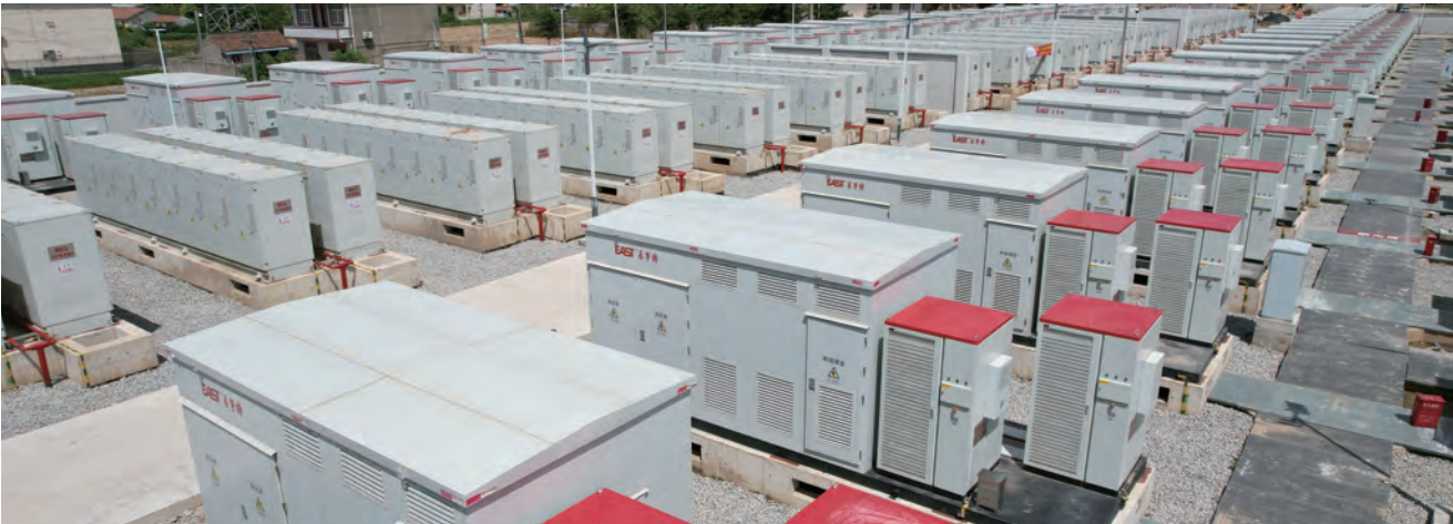
155MW/369.52MWh East Qidong Energy Storage Power Station
