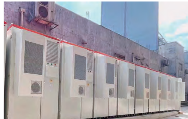
1.4MW/3.01MWh User-side energy storage of Yiquan Science and Technology Park
