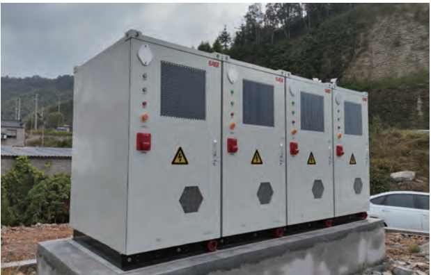
540kW/1044kWh Wuyi County Jintong Heavy Truck Fast Charging Station Energy Storage Project
