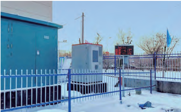
2.9MW/6.23MWh Xinjiang Yining Optical Storage, Charging, Swapping and Discharging Integrated Project
