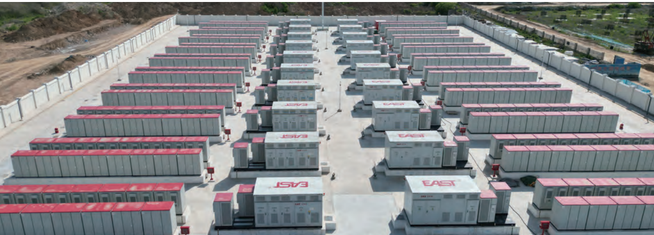
50MW/100MWh Shared Energy Storage Power Station in Hubin District, Sanmenxia City
