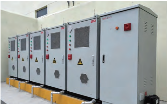
675kW/1305kWh Suqian Yike Xuyang Feed Energy Storage Project
