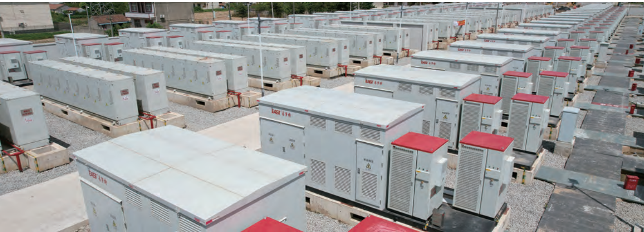
155MW/369.52MWh East Qidong Energy Storage Power Station
