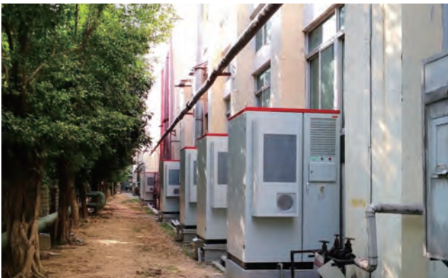
700kW/1505kWh Commercial and Industrial Energy Storage Project of Guangzhou Yuekang Biopharmaceutical Co., Ltd.
