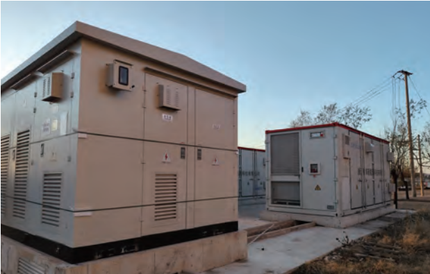
10MW/20MWh Chiku New Energy Tangshan User-Side Energy Storage Project
