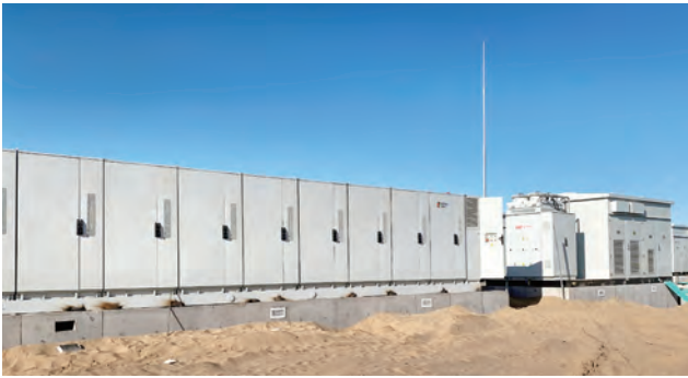
40MW/80MWh Energy Storage Supporting the 100MW Photovoltaic Sand Control Project in Dengkou County, Inner Mongolia, SPIC
