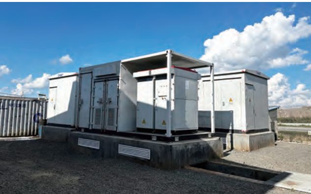
3.5MW/10MWh Huayou Cobalt's Grid-Forming Energy Storage Project at the Lukuni Plant in the Democratic Republic of the Congo
