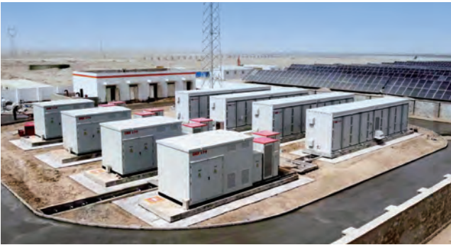
10MW/20MWh Energy Storage Supporting the 100MW Photovoltaic Power Generation Project of Trina Solar in Yuli County, Bazhou
