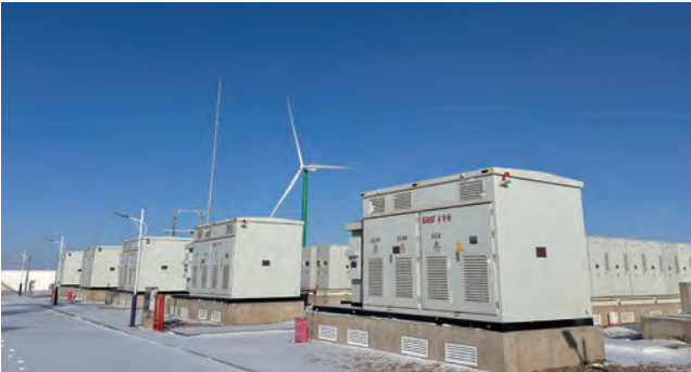
15MW/60MWh Zhangye Linze Banqiao North BeachPhase I 100MW Wind Power Project with Energy Storage
